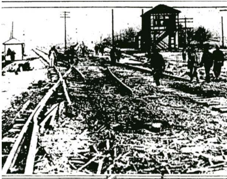
Worthington interlocking tower, where cleanup from a broken rail caused derailment continues. The camera is pointed north looking down the Big four right-of-way. The Pennsy's double tracked Sandusky Branch is crossing the Big Four. There is not much left of the diamond.
